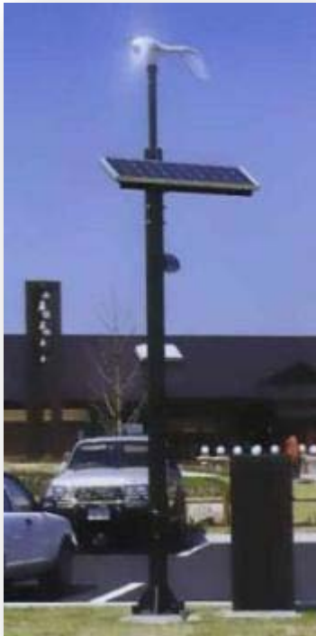
Hybrid Street Lighting
