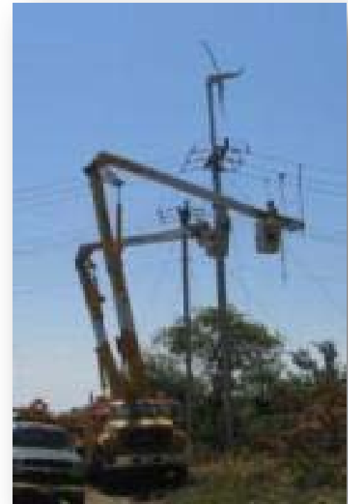
Utility Power Pole Integration
