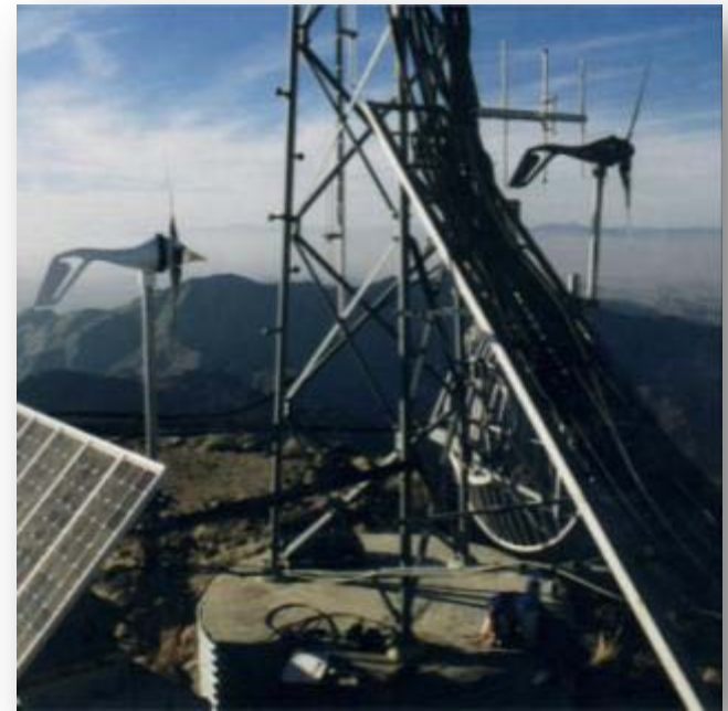
Remote Telecom Electrification
